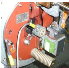
Picture two: An encoder is mounted on a stepped shaft extension inside the brake enclosure. The encoder is tethered to the brake support plate.
